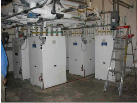
Ground source heat pumps at Harvard
