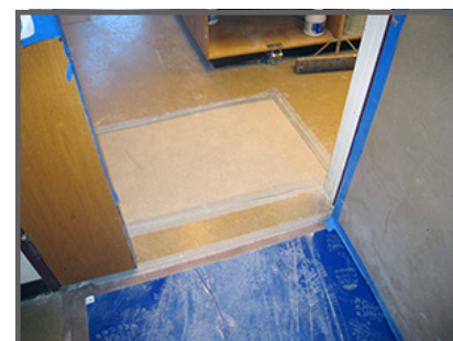
IAQ Management Housekeeping: Walk-off mats at entrance
